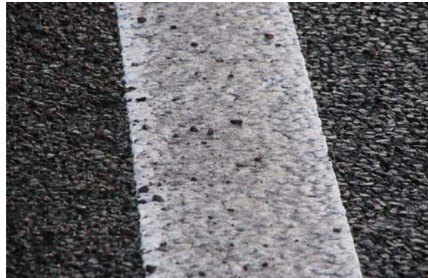
Figure 3.2 – Loose aggregate on the pavement surface due to raveling.
