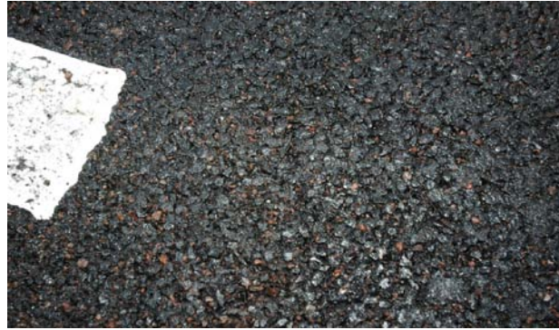
Figure 3.4 – Pavement surface in un-trafficked areas prior to replacement.
