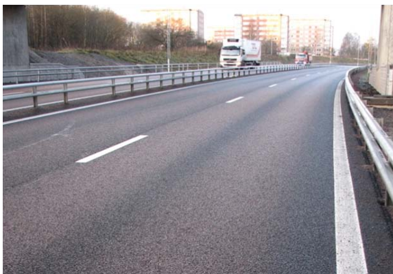
Figure 3.1 – Pavement surface prior to replacement.
