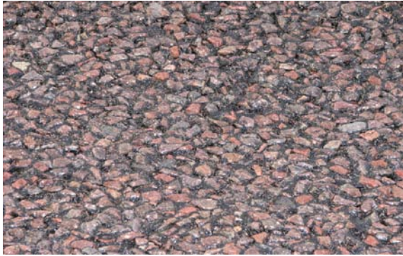
Figure 3.3 – Pavement surface in trafficked areas prior to replacement.
